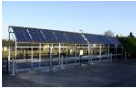
CAFRE, UK (Dairy Cow Unit of 140 cows) Collectors' area: 22 sqm Storage capacity: 1200 L (Domestic Hot Water)
