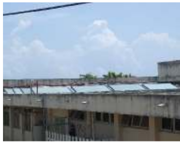
St' Ann's Bay Hospital, Jamaica Collectors' area: 40m 2 Storage capacity: 5600 L (Domestic Hot Water)
