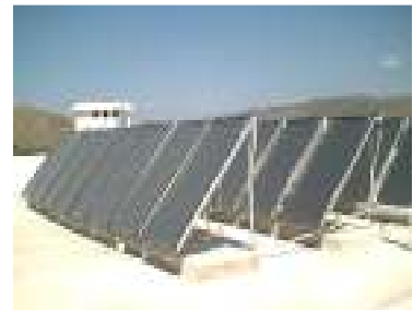
Hotel in Karistos, Greece Collectors' area: 60m 2 Storage capacity: 3 m 3 (Domestic Hot Water + Pool heating)
